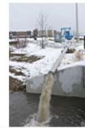
Pumping water out of Fargo, ND, April 1, 2009, at the rate of 6,500 gallons every 10 minutes. Photo by Patsy Lynch/FEMA.
