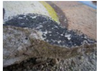
Section of fallen wall shows how thin the original paint was applied directly to the concrete wall
