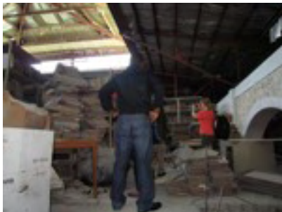
The building of the National Archive seems sound but roof structure has been partially damaged
