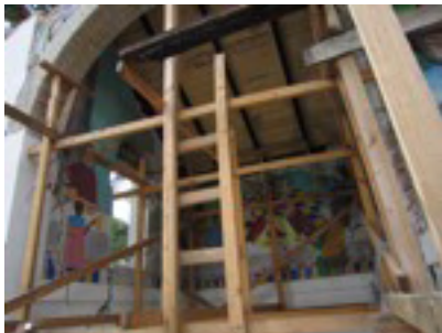
Wooden beam is just supporting archway and not the mural image wall
