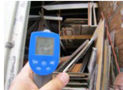
inside roof temperature was 105 F
