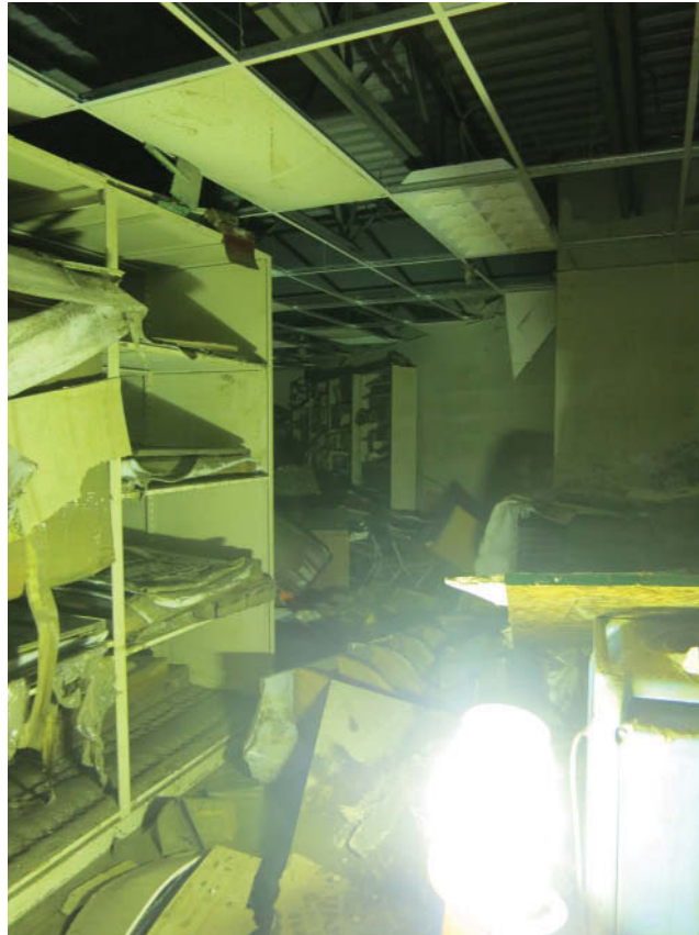
Fig. 6. First glimpses of the state of the off-site storage. Courtesy of Irene Kerr.
